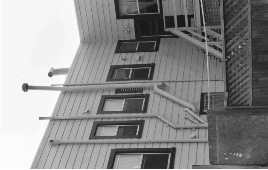
2340 Lane Street: External plumbing, deteriorated fence.
