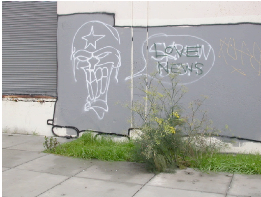
Illinois Street between Cesar Chavez Street and Marin Street: Graffiti, deteriorated cement, weeds encroaching on sidewalk.
