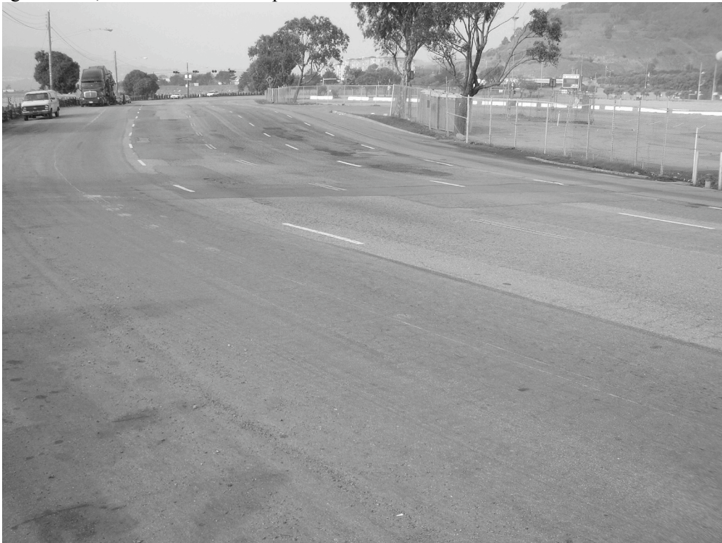
Hunters Point Expressway, east side of Candlestick Park: Lack of sidewalk, uneven, deteriorated pavement and deteriorated fence.
