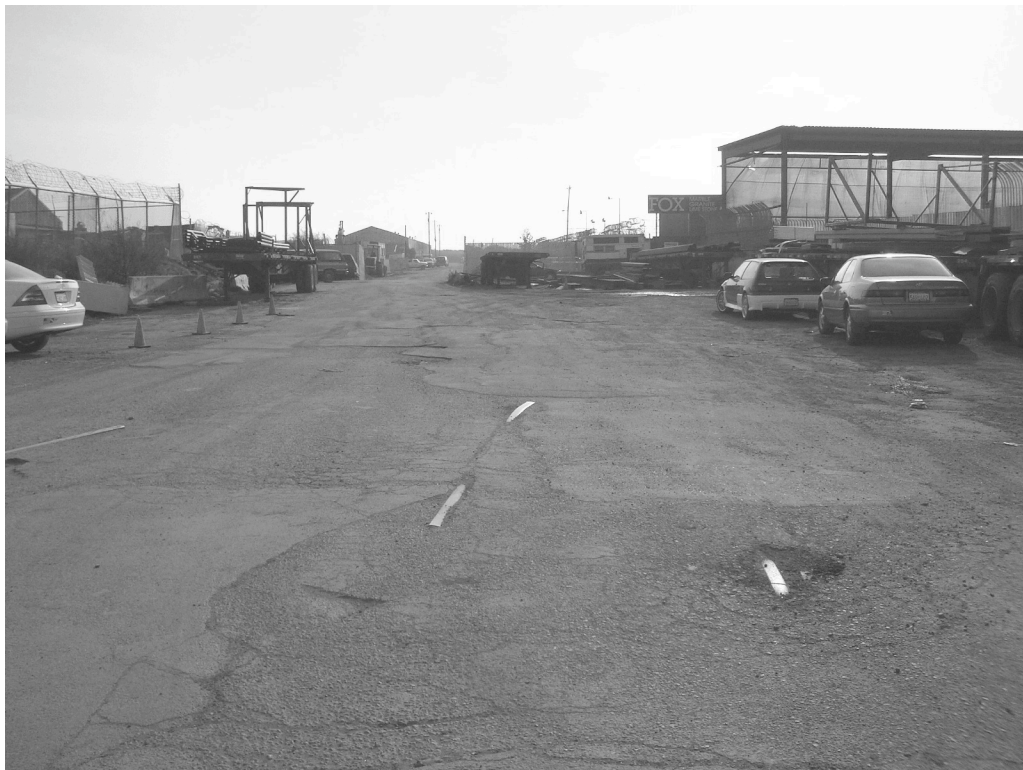
Armstrong Avenue at Ingalls Street, to the Southeast: Deteriorated, uneven pavement over abandoned railroad tracks.
