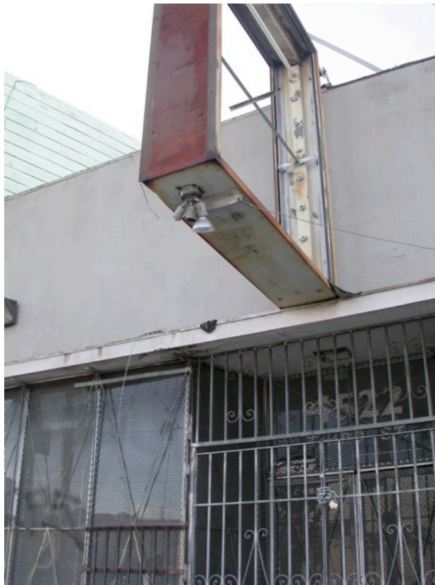
4522 Third Street: Vacant retail building and deteriorated signage.
