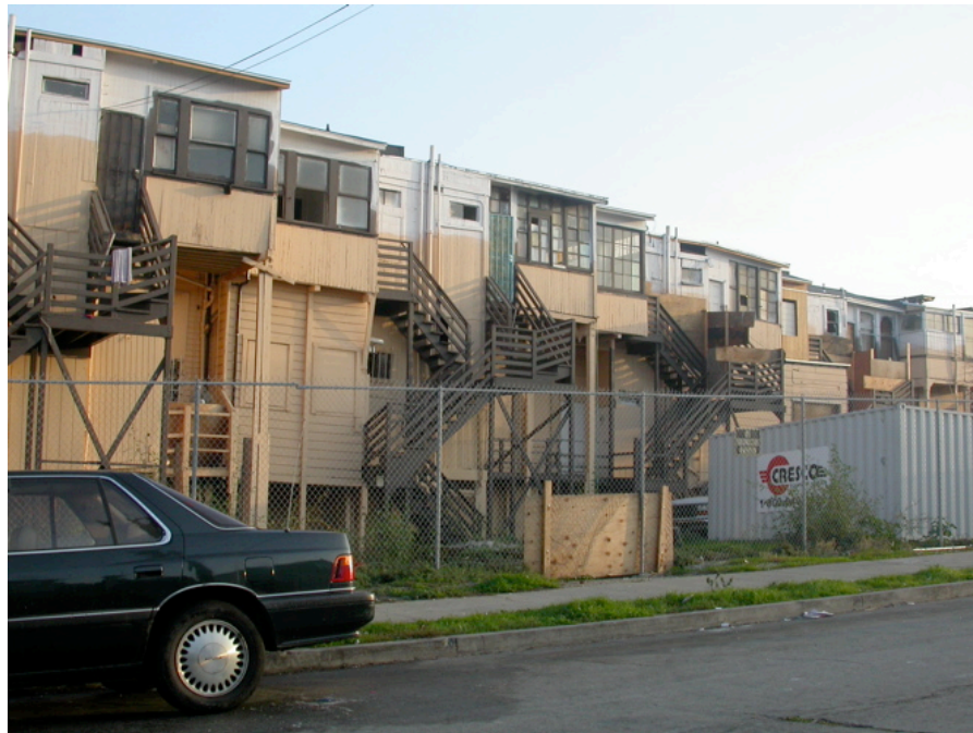
Back of 3rd Street on Newhall Street: Dilapidated structures, substandard construction, unsound egress, deferred maintenance, missing gutters, deteriorated windows.
