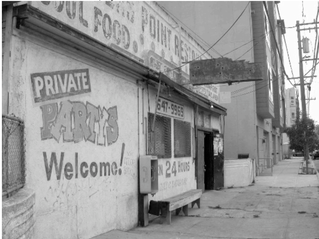
840 Innes Avenue: Extensively deteriorated building, faded and peeling paint, deferred maintenance, graffiti, dilapidated signage, missing gutters and downspouts, mold, cracks in front façade, poorly maintained sidewalk, faulty wiring.
