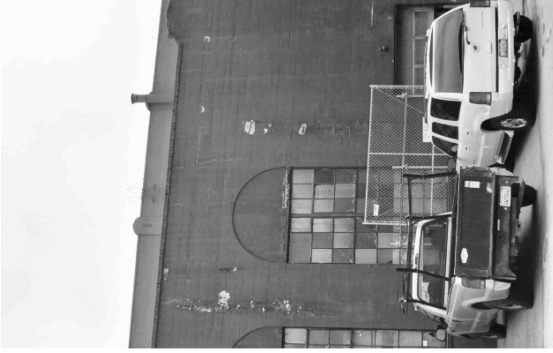
1485 Bayshore Blvd (Rear): Extensively deteriorated concrete wall, chipped paint, deteriorated windows.
