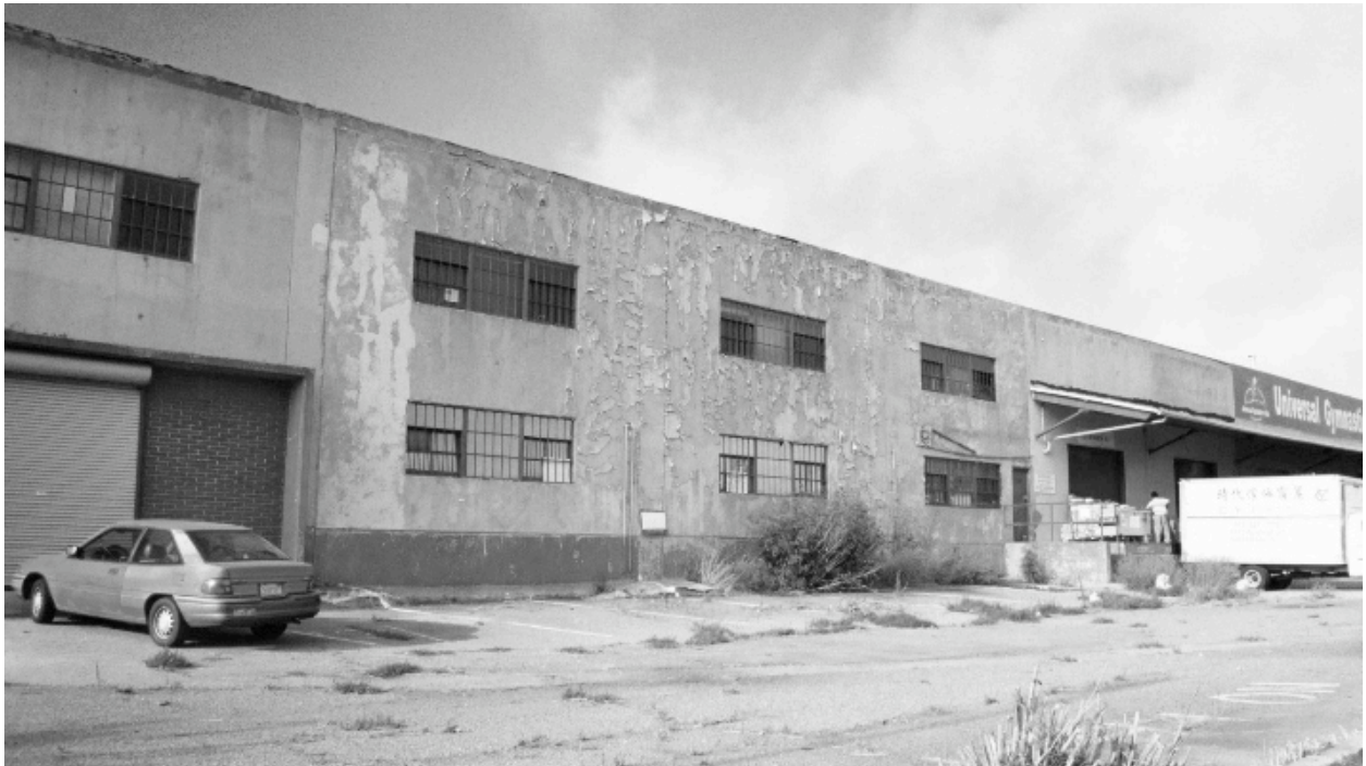
1398 Marin Street (Rear): Deteriorated building, peeling paint, deferred maintenance, deteriorated pavement, poorly maintained landscaping.
