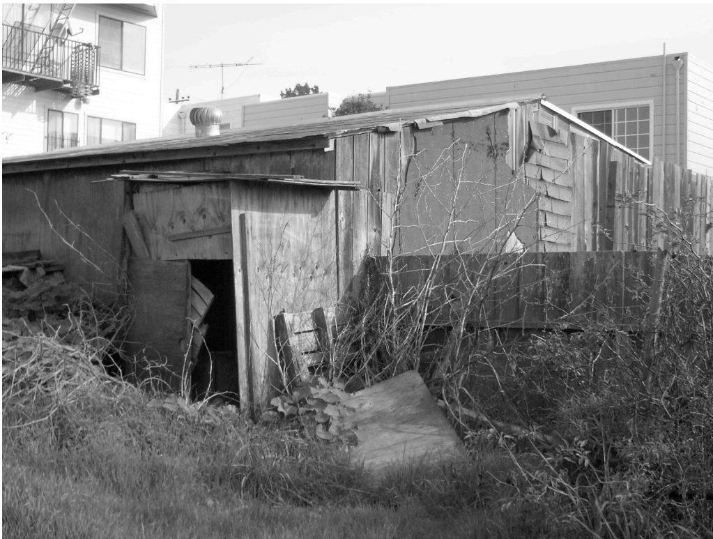
331 Thornton Avenue (Rear): Unsafe dilapidated shed, missing and deteriorated siding materials.
