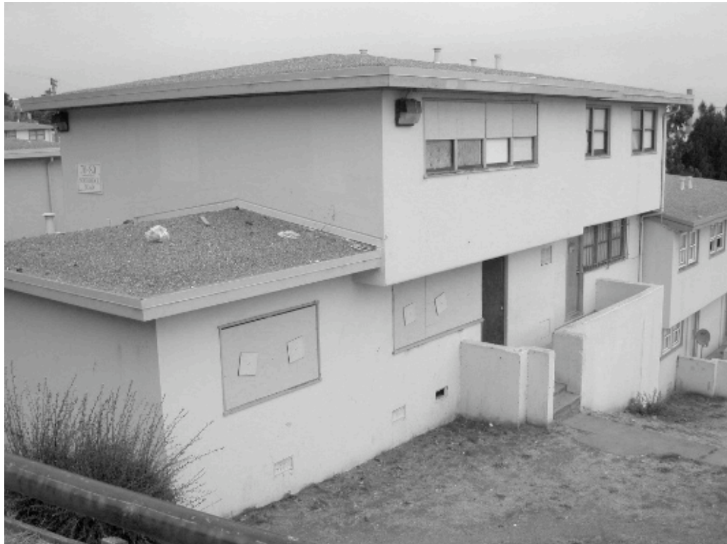
70-80 Northridge Road: Deteriorated building, partially vacant, boarded-up windows, trash accumulation on roof, dry rot on window frame.
