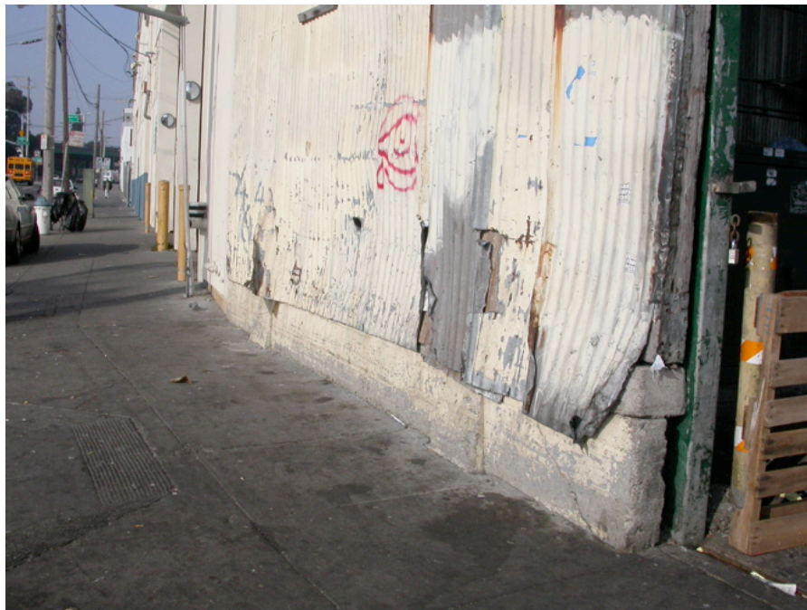
2380 Jerrold Avenue: Deteriorated, rusted corrugated steel siding. [Detail of building in above photograph]
