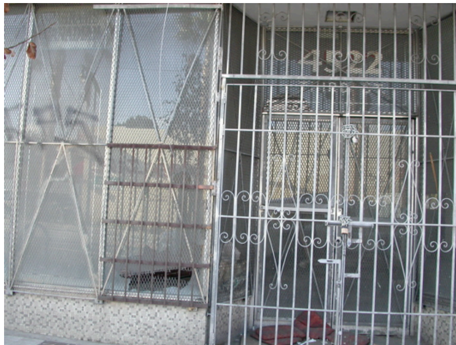
4522 Third Street (detail of building as above): Vacant commercial building, broken window, and graffiti.
