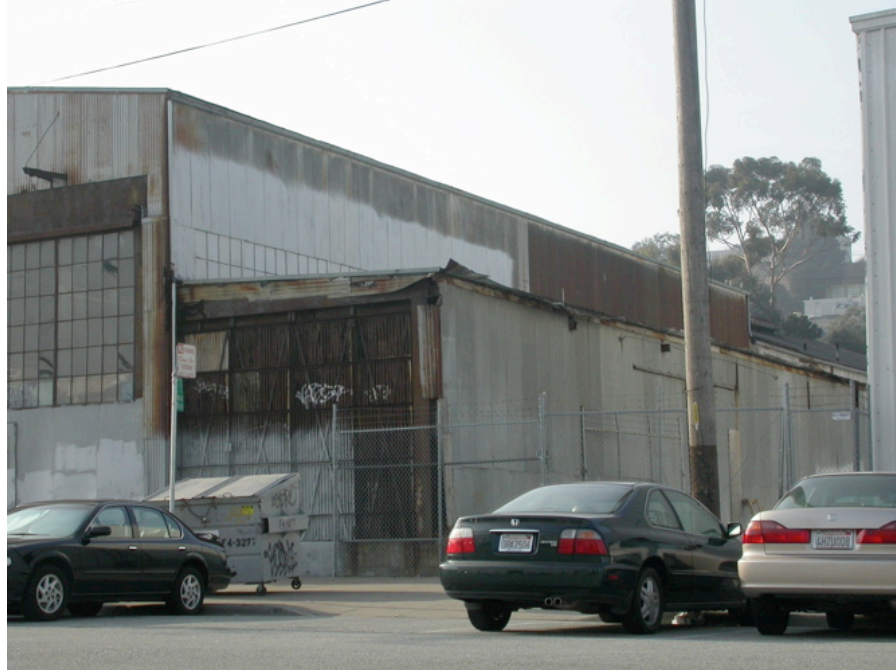
235 Bayshore Boulevard: Dilapidated structure, sagging and partially missing siding, extensively deteriorated and rusted roof, missing gutters on small structure, deteriorated windows.
