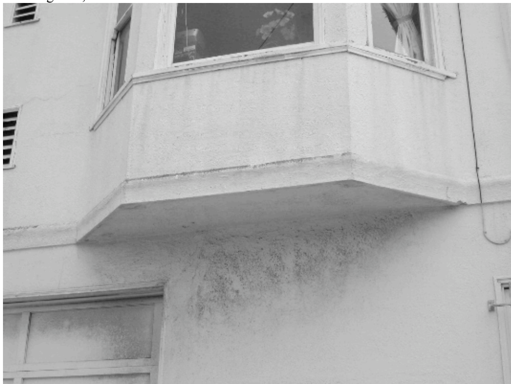
Northeast corner, Gilman Avenue and Jennings Street: Water damage and mold underneath bay window, chipped paint, cracks in stucco.
