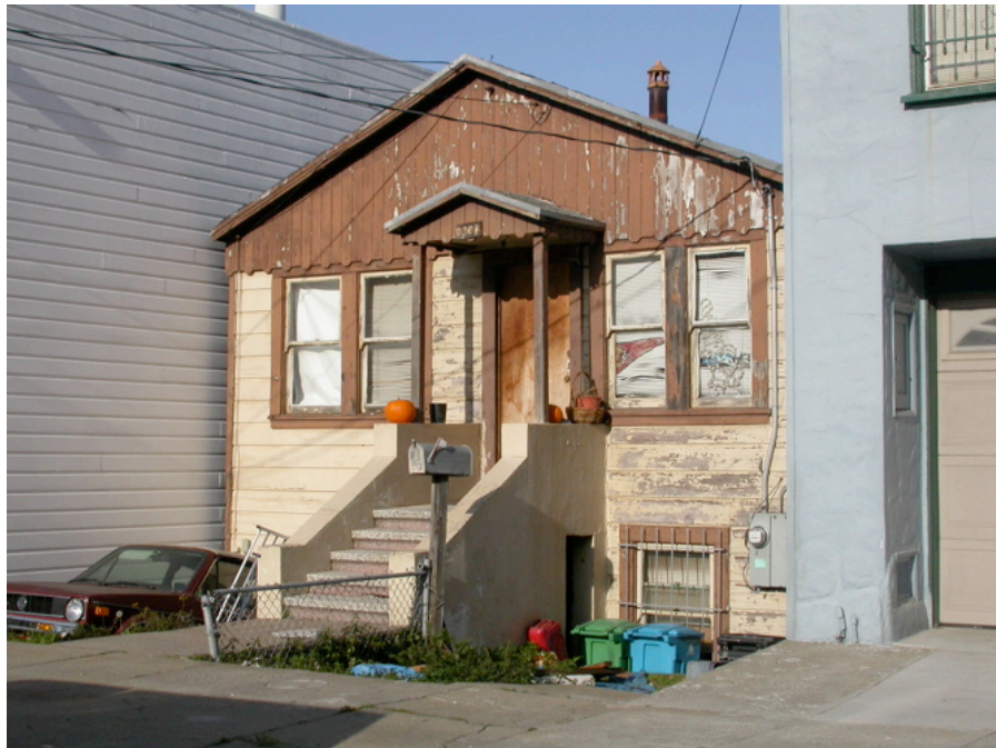
1030 Jamestown Avenue: Dilapidated residence, deferred maintenance, and deteriorated painting.
