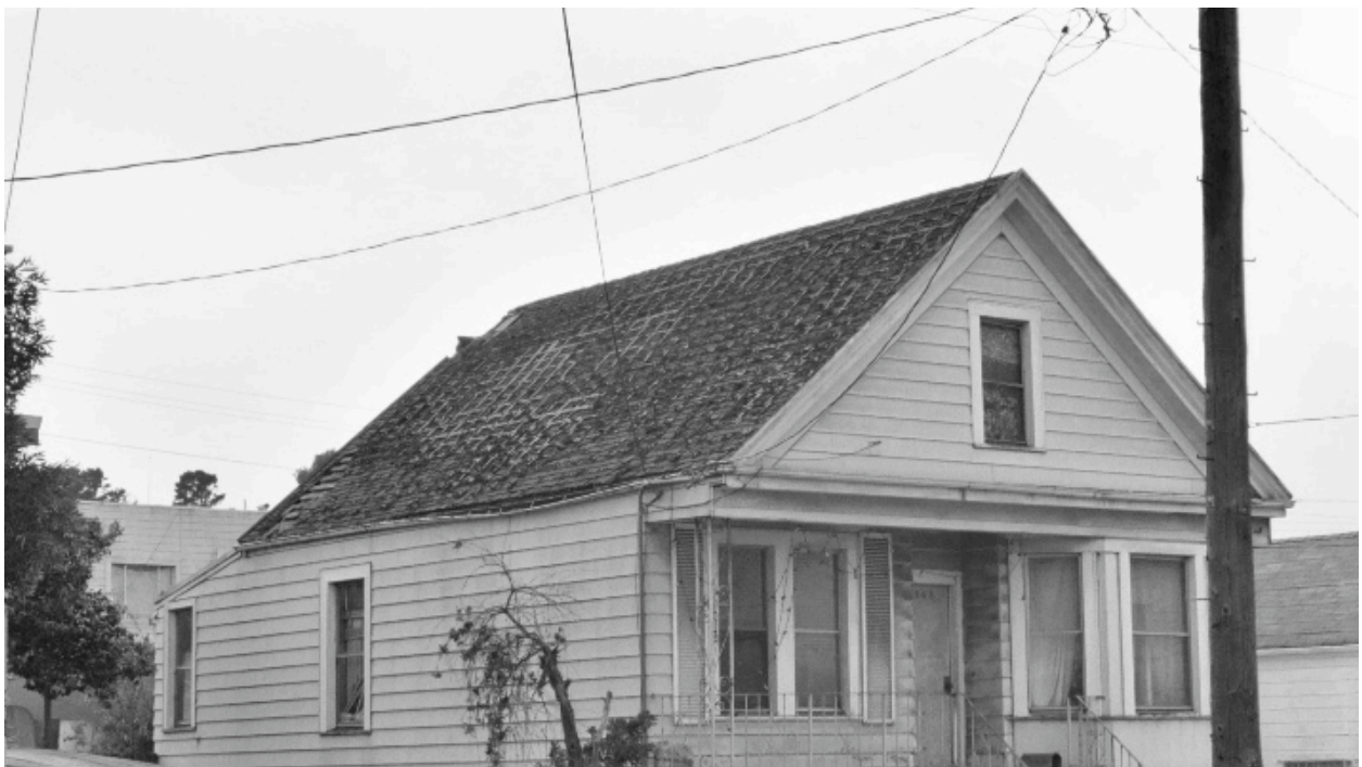
1963 Oakdale Avenue: Dilapidated roof, sagging and deteriorated gutters, missing downspouts.
