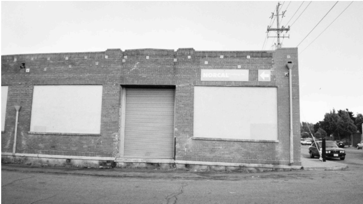
Northeast corner of Quint Street and Evans Avenue: Partially reinforced masonry building, deteriorated masonry, alignment problems, boarded-up windows, lack of sidewalk, deteriorated pavement.
