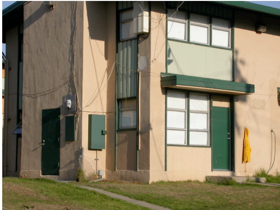
78 Nichols Road (Alice Griffith): Faulty wiring.
