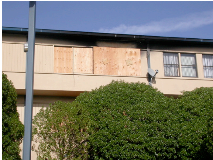
1114 - 1124 Palou Avenue (Hunters Point SFHA Development): Fire damage, boarded windows, apparently vacant residence.
