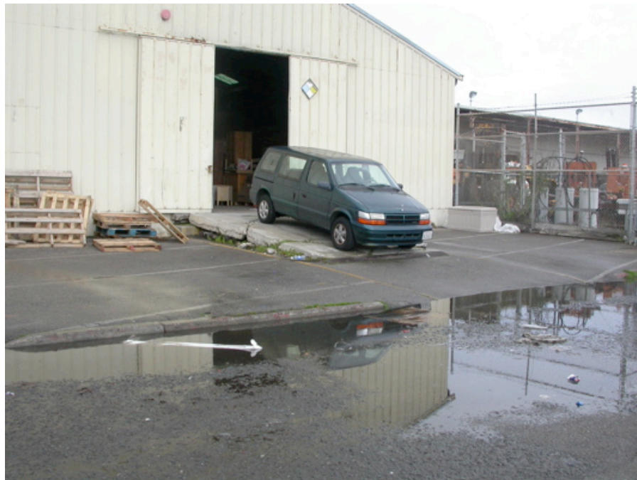
888 Marin Street: Standing water indicating potential inadequate drainage, cracked pavement on delivery ramp.
