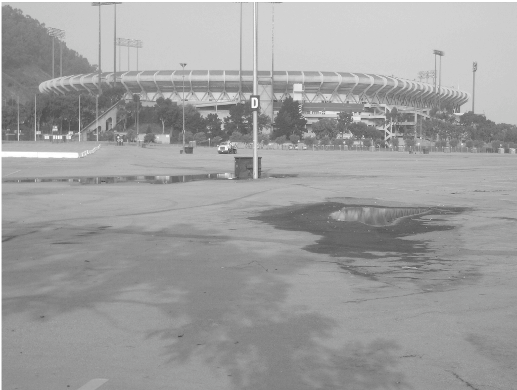
East side of Candlestick Park: Uneven, deteriorated pavement, standing water.
