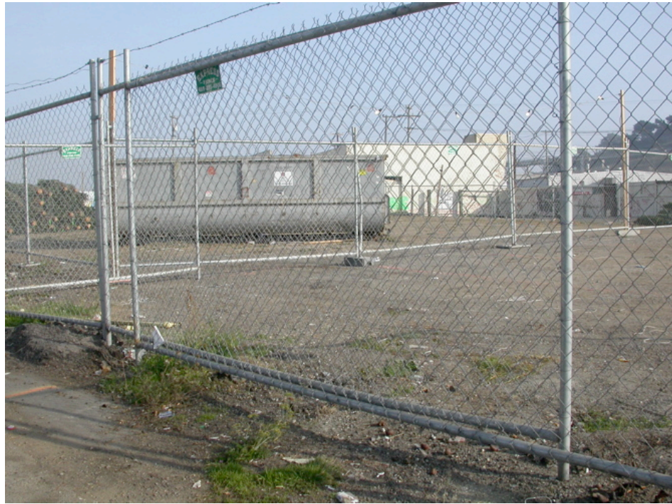
Northeast corner, Bayshore Boulevard and Industrial Street: Large, vacant and underutilized lot, cracked and deteriorated concrete pavement.
