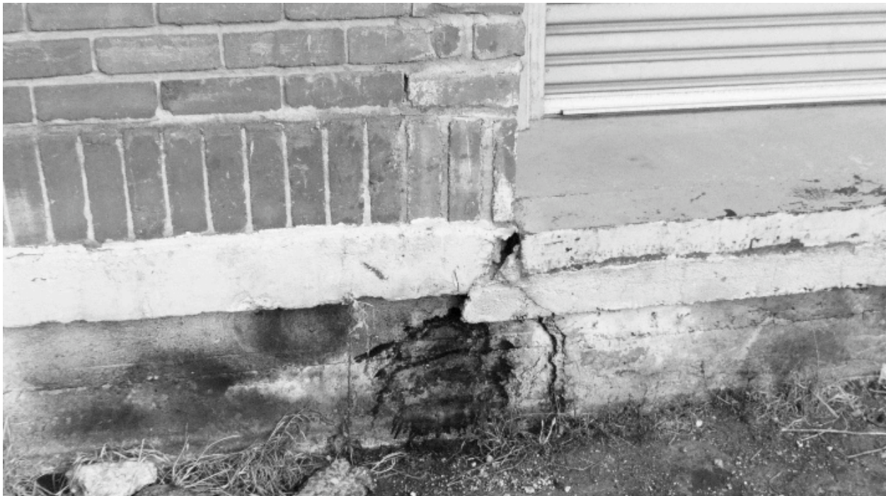
Northeast corner of Quint Street and Evans Avenue: Large, unsafe crack where masonry wall meets building foundation, deteriorated masonry, mold. [Detail of building in photograph above]
