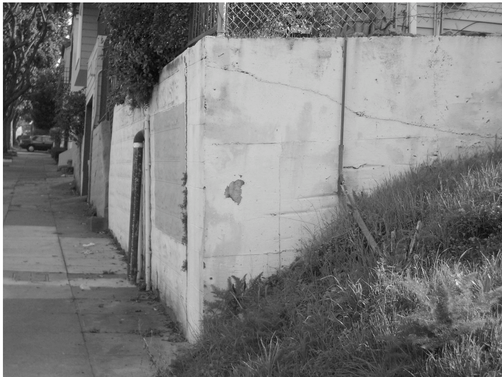
Southeast corner, Mendell Street and Hudson Avenue: Deteriorated, cracked retaining wall.
