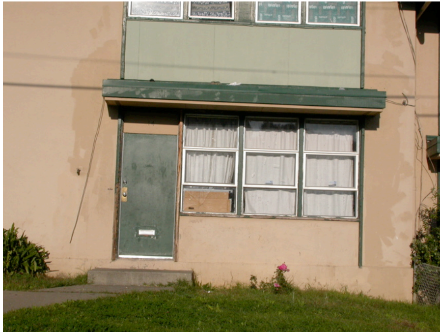
14 Cameron Way (Alice Griffith): Dilapidated residence, broken window, deferred maintenance and faulty wiring.
