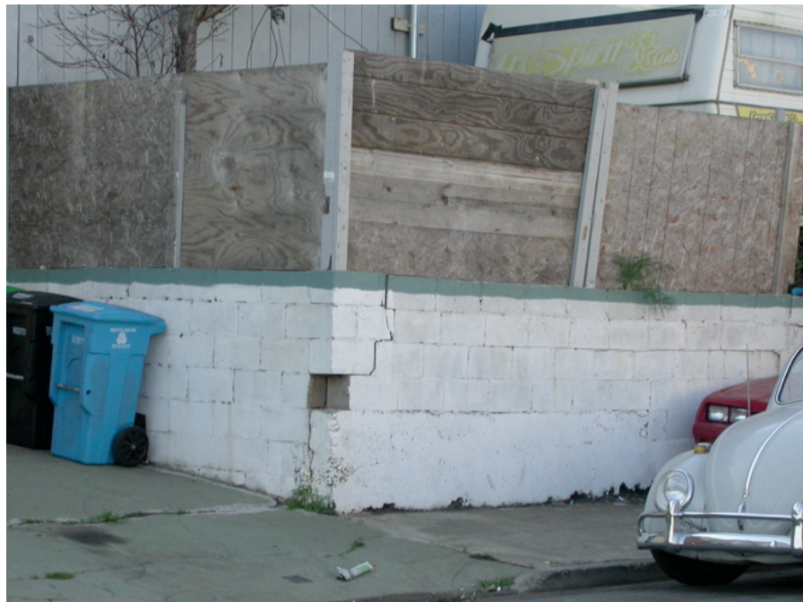
2901 Hawes Street: Retaining wall with large, unsafe crack, cracked and deteriorated sidewalk, informal and substandard fencing. [Detail of wall and sidewalk in photograph above]
