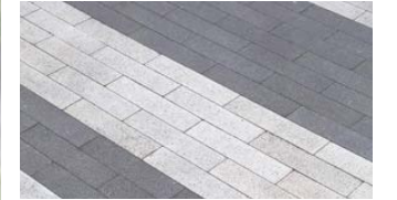
2 Basalte 6\"X12\" or Hexagon Concrete Unit Pavers In Two Colors With Ground Face Finish In Stacked Bond With Linear Pattern Per Plans
