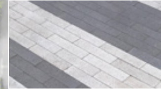
2 Basalt 6"X12" or Hexagon Concrete Unit Pavers In Two Colors With Ground Face Finish In Stacked Bond With Linear Pattern Per Plans
