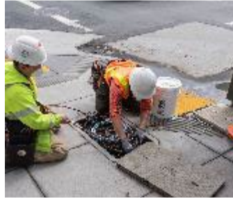
Existing Electrical Power
